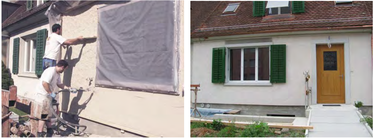
Figure 18: Renovation of an old row house in Winterthur: spraying and equalizing of aerogel render (left), aerogel render before application of finishing render
