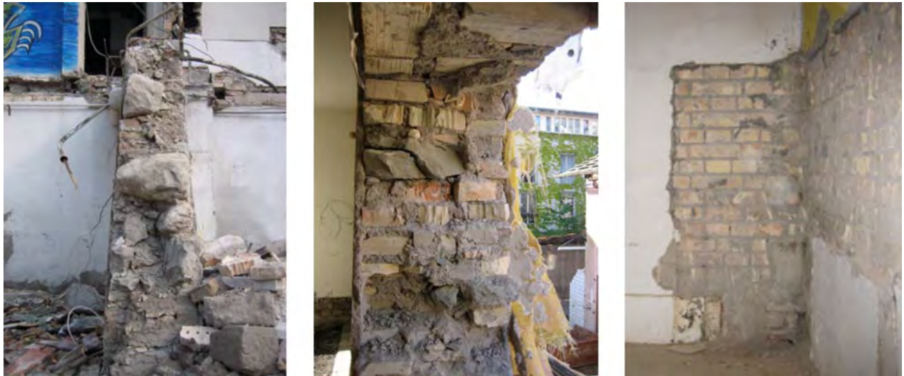
Figure 4: Typical wall constructions: natural stone wall (Seefeldstrasse), mixed masonry wall (Feldegstrasse), brick wall (Kernstrasse)
