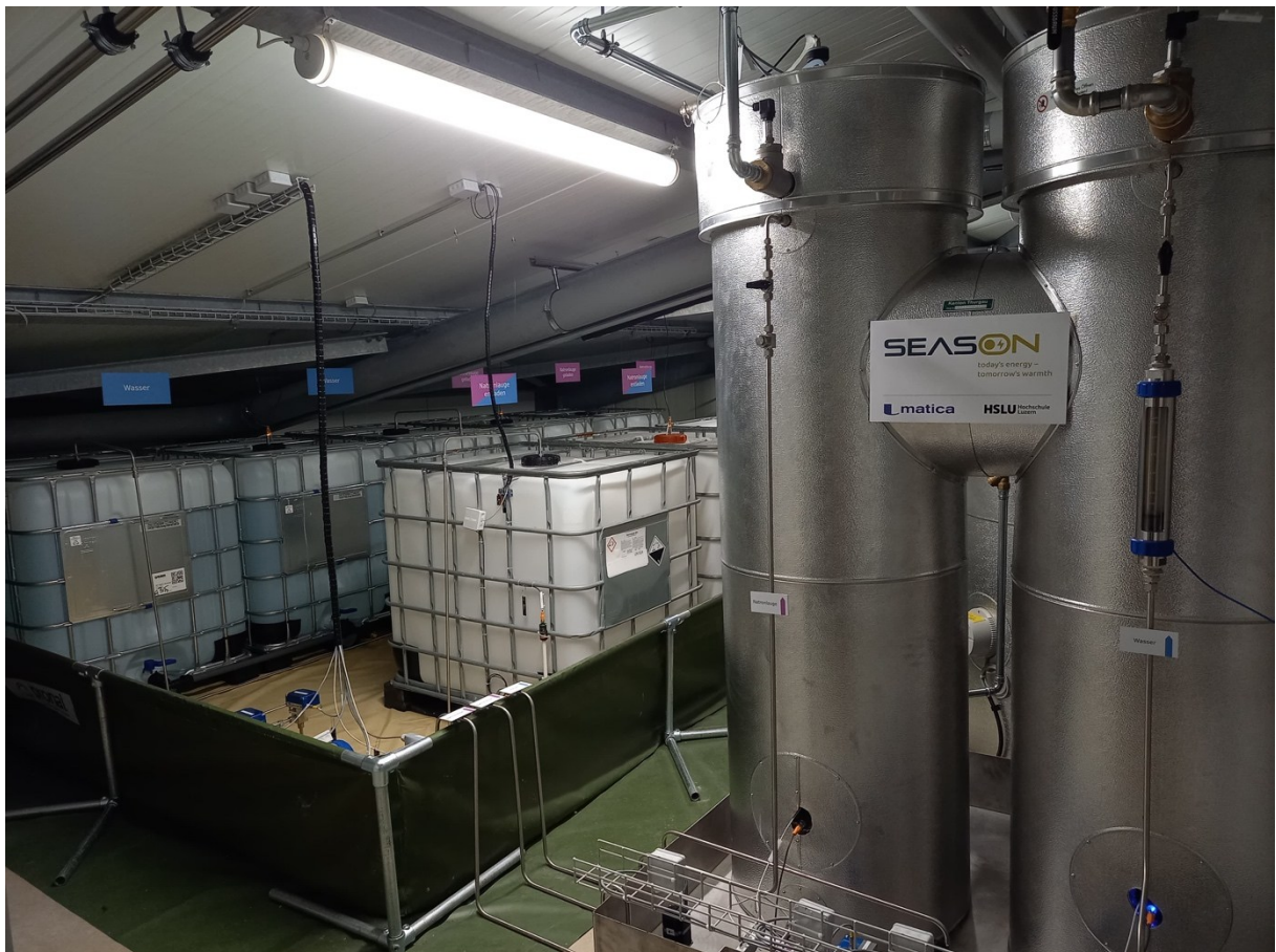
Image of the Sorption Storage Heat Pump installed in Frauenfeld. On the right is the heat and mass exchanger, while the sorbent storage is on the left. The two components are connected by stainless steel pipes, valves, and pumps. Source: HSLU, 2024.
