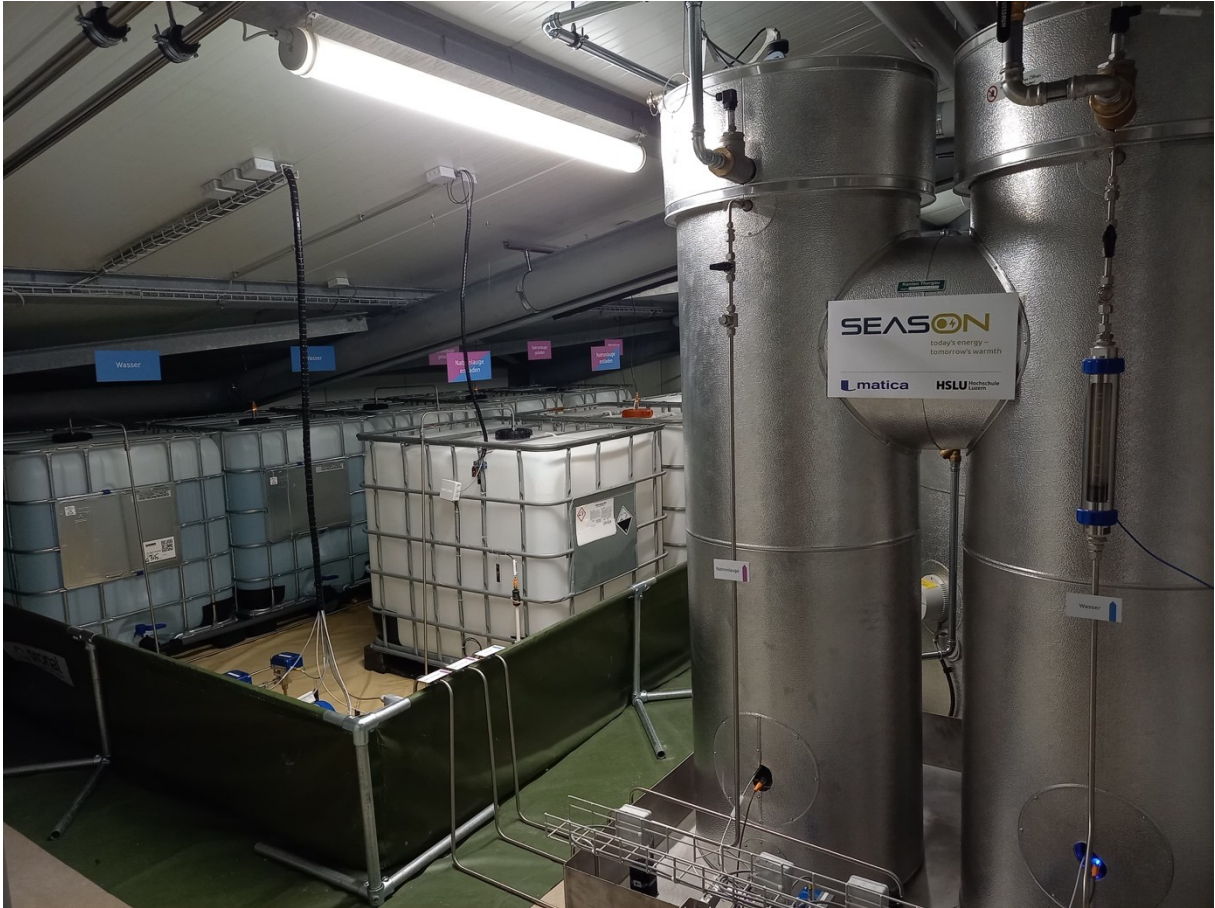
Figure 11: Photo of the complete system installed in Frauenfeld. On the left back are the working pair tanks and on the right front is the heat and mass exchanger. In this picture version HMX-1.
