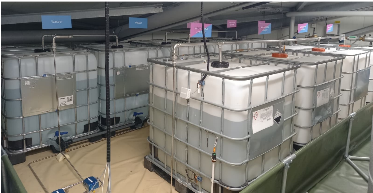
Figure 9: Picture of the installed absorbent and absorbate tanks. Three tanks hold concentrated aqueous sodium hydroxide and two hold water, in charged state, and four hold diluted aqueous sodium hydroxide in discharged state. This amounts to a storage capacity of around 1MWh, depending on the discharging process.
