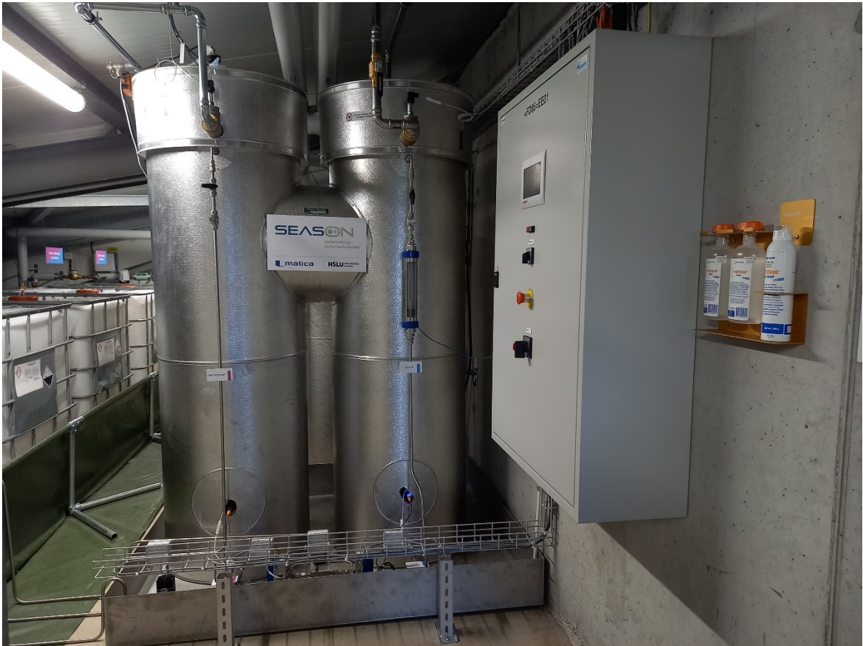
Figure 15: Image of the HMXv1 system installation in Frauenfeld. Front right is the HMX and left back the storage tanks in the safety basin. The two are connected with stainless-steel tubes.
