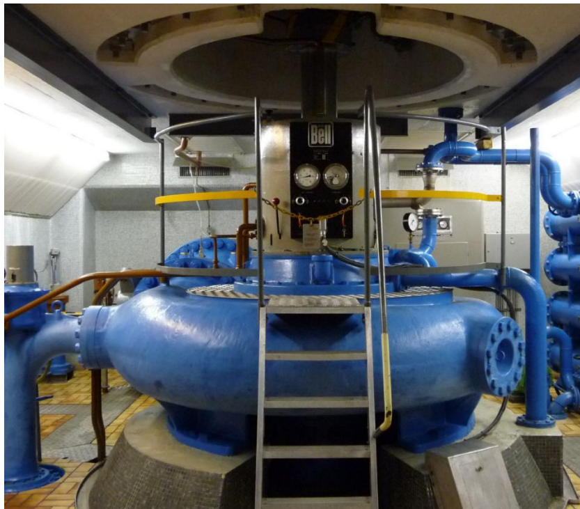
Figure 23: non-regulated Francis turbine equipping the power plant of KW Altstafel (source: HES-SO).
