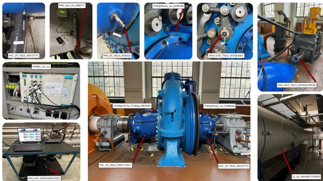
Figure 77 : Photographs of existing and temporarily installed sensors at KW Mörel.
