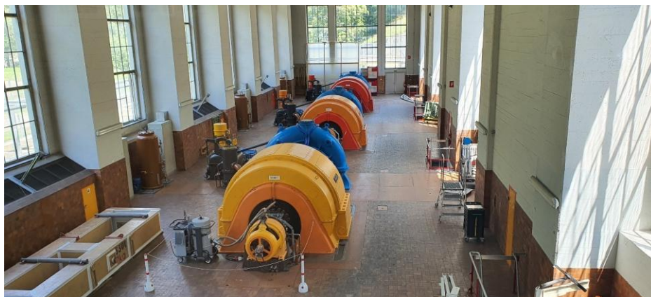
Figure 18: View of the three double-Francis units of the Mörel hydropower plant.
