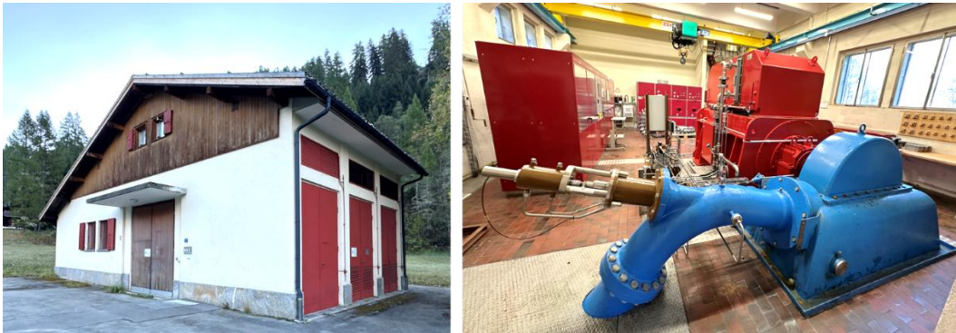
Figure 22: Outside and inside views of the KW Merezenbach hydropower plant.
