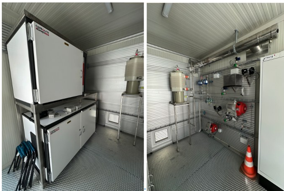
Figure 69. Membrane skid for testing graphene membranes for the separation of flue gas from combined heat and power (CHP), installed in Aigle under the premises of GAZNAT.
