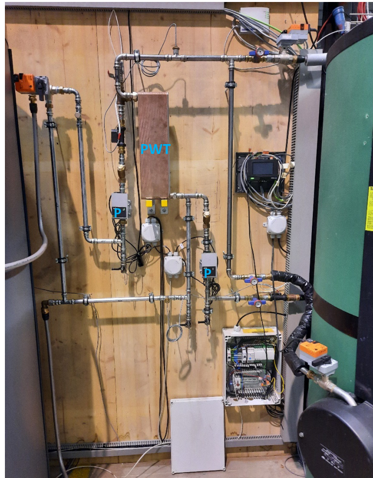
Figure 2: Storage transfer station with plate heat exchanger (PWT), circulation pumps (P) and valves (orange).
