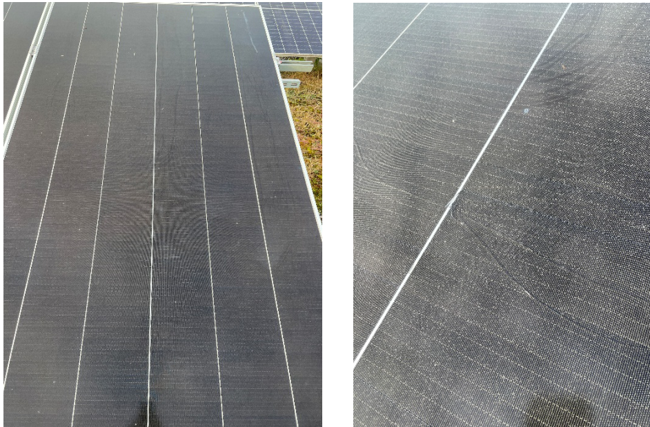
Figure 30: Whole-of-module view of broken module #14 (second module breakage in this position, left), and detailed view on glass crack (right).
