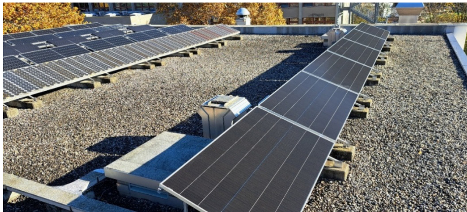
Figure 7: Five new technologies were installed near the 40+ years old PV system TISO on Aula Magna roof in Campus Trevano.
