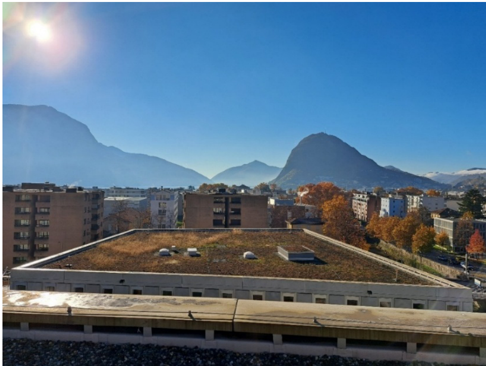
Figure 1: View of the South roof looking West, from the USI/SUPSI building to the East, before the PV system was installed. Note the objects on the roof which constrain the degrees of freedom for array placements. The building from where the photograph was taken causes shading of the South roof.
