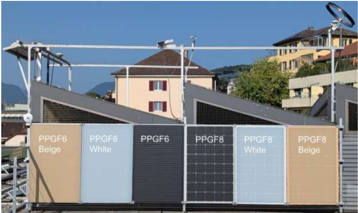
Fig. 38 Demonstrator site on microcity rooftop at Neuchâtel, Switzerland
