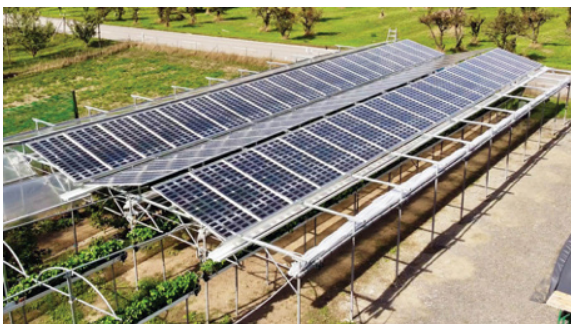
Figure 12: Photographs of the projects based on the GEN2 agrivoltaic solution in Conthey. Left: 16kWp GEN2 demonstrator. Right: 265kWp commercial-scale GEN2 installation with dedicated areas optimized for the cultivation of raspberries and strawberries.
