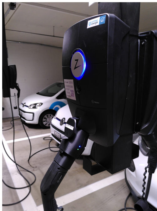
Figure 7. Deployed plug adapter with charge controller at an EVSE in Münchenstein.
