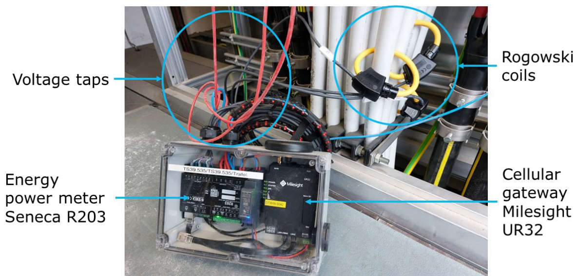
Figure 12. Mobile grid measurement unit installed at the level 6 transformer in Münchenstein.
