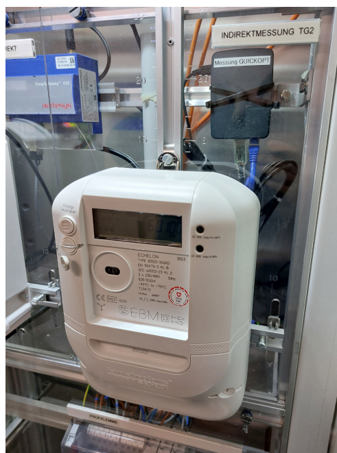
Figure 10. Smart meter monitoring in Münchenstein with EnergyX device in the background.
