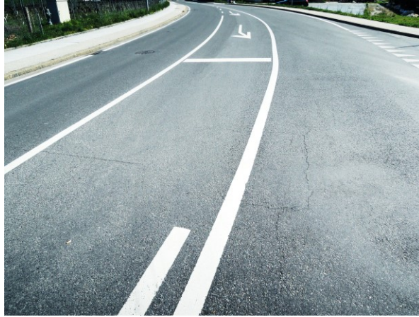
Figure 30: Cracks at the intersection of turning lane in Section B
