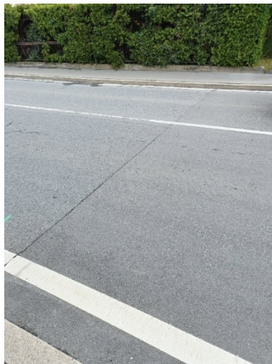
Figure 31: Construction joint crack at Section A
