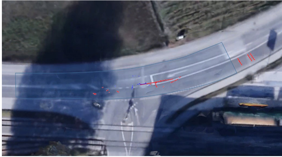
Figure 23: Crack situation in Section B
