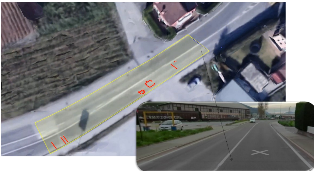
Figure 22: Crack situation in Section A
