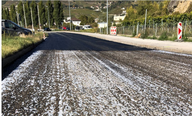
Figure 8: Stone chipping on one of the reinforcement sections
