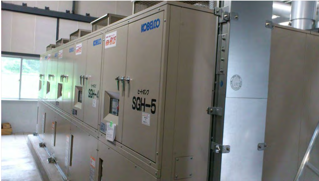
Figure 1: External appearance of heat pump units (5 units integrated)
