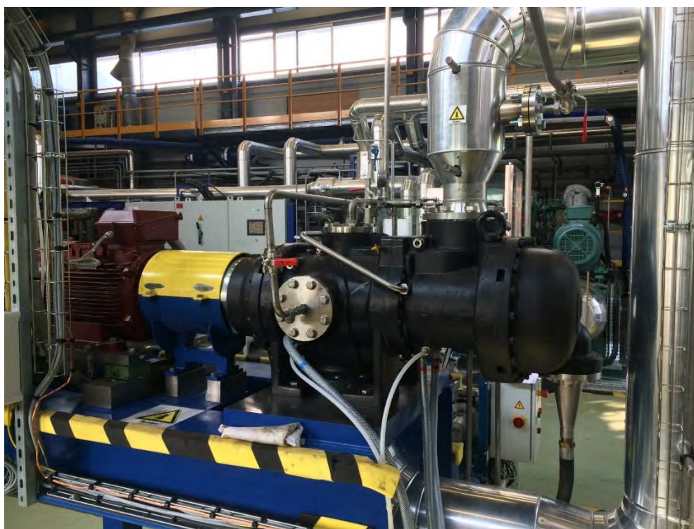
Figure 1: SRM prototype compressor skid
