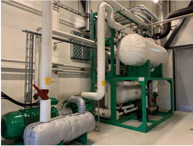
Figure 2: GreenPAC heat pump at Tine Bergen.
