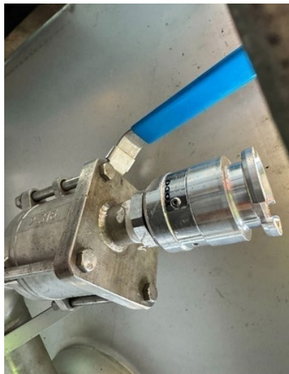
Figure 16: Methanol safe transfer connection
