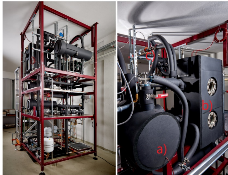
Figure 13: Test facility at TU Berlin, a) evaporator, b) absorber, c) expansion machine [5].
