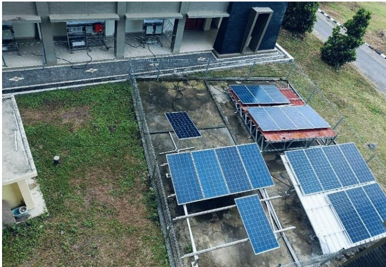
Solar PV equipment in BPVP Lombok
