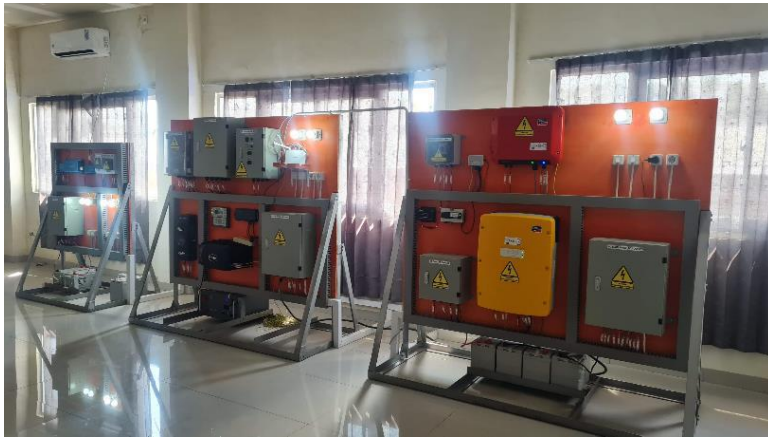
Polytechnic Makassar, solar PV lab modules
