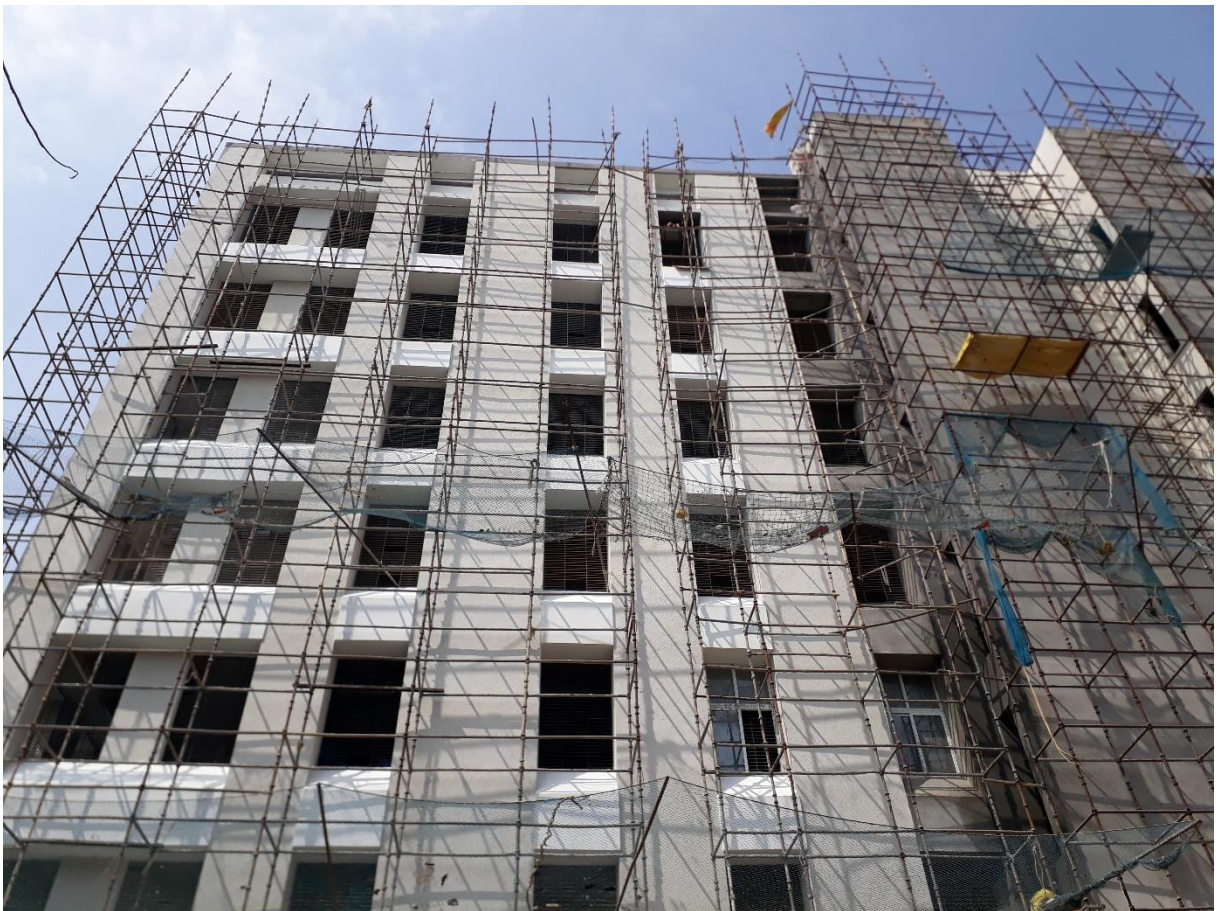
Construction site in Chennai (Madras), India, one of the participating countries in IEA EBC Annex 89
