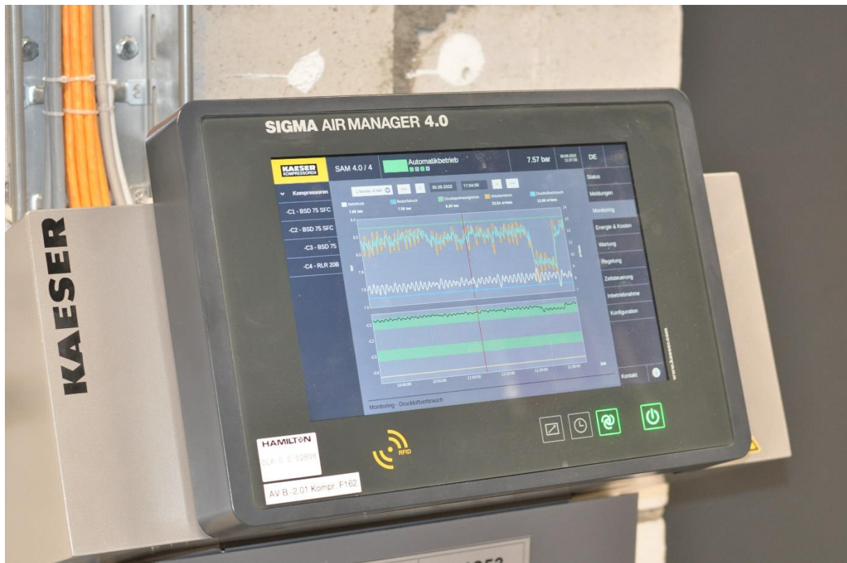
Figure 1 The newly installed air pressure management system of the first good example, SIGMA 4.0 (photograph: Pascal Kienast)
