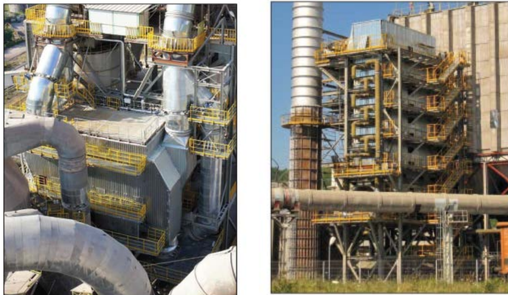
Figure 19. Preheater heat exchanger (left) and clinker cooler heat exchanger (right) [55].
