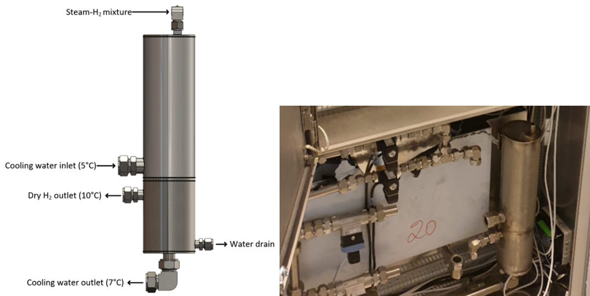
Figure 25: Condenser to dry the produced hydrogen (left: CAD part, right: the condenser mounted on the BoP)
