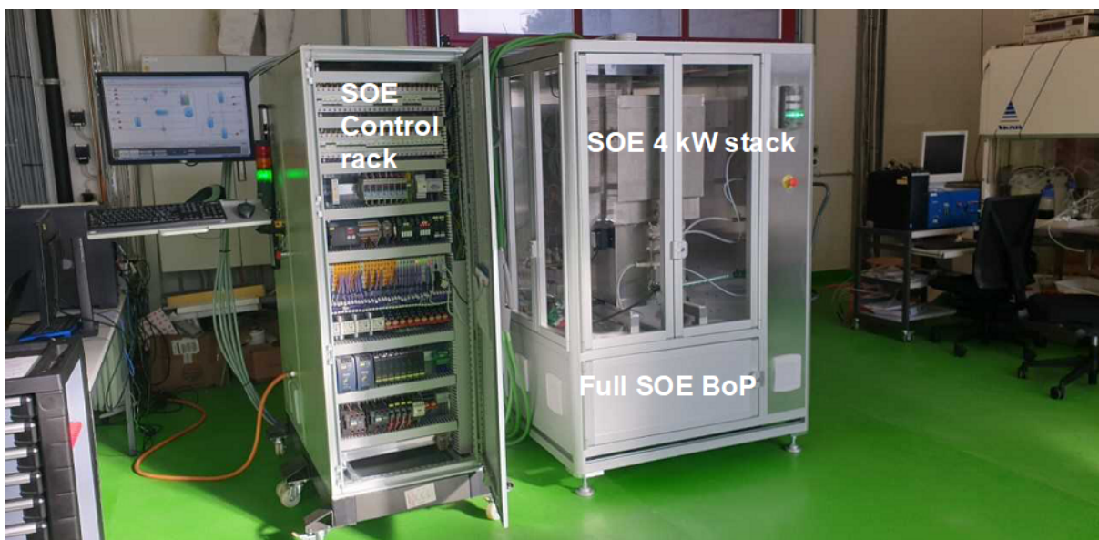
Figure 23: The SoE-BoP and the control rack prepared by EPFL, before being moved to the Research Platform Power-to-X at OST.
