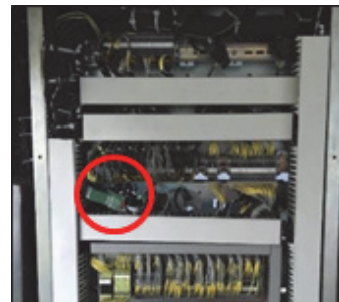
Fig. 5: Current sensor in the driver's cabinet
