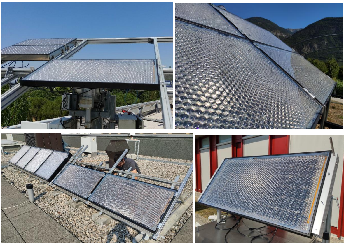
Figure 31: Insolight modules installed at UPM in Madrid (top-left), Conthey (top-right) and at EPFL in Lausanne (bottom).
