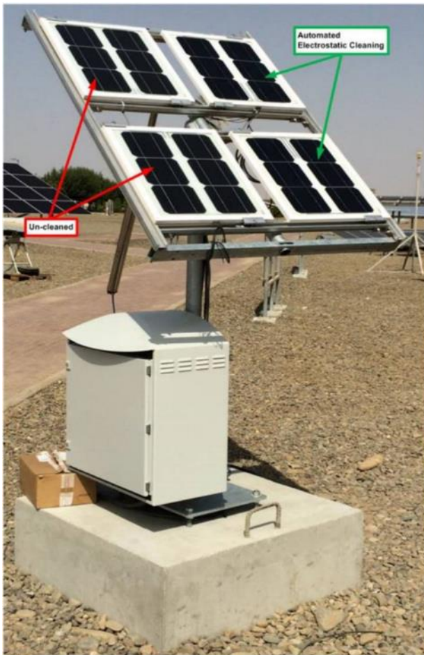
Fig. 4.25. Pilot field test of the electrodynamic cleaning system (EDS) from CleanFIZZ at KAUST (King Abdullah University for Science and Technology) near Jeddah in Saudi Arabia.
