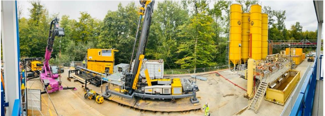
Figure 26: Status today with the drilling rig and the supporting infrastructure being placed, in final preparations for acceptance of the unit.
