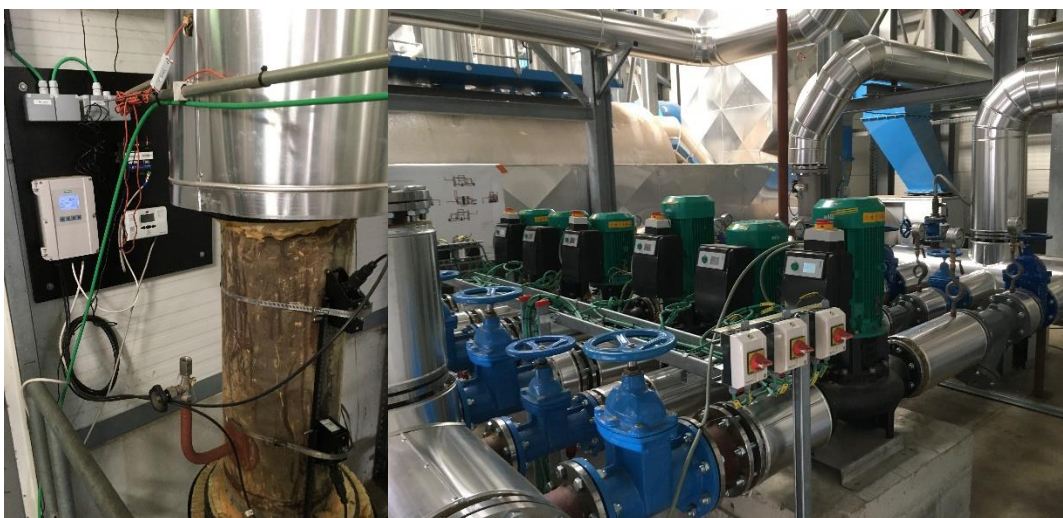
Figure 5: Left: Installation of an ultrasonic flowmeter, heat meter with IOT gateway on a DN250 DHN pipe. Right: New substation for the residential area.
