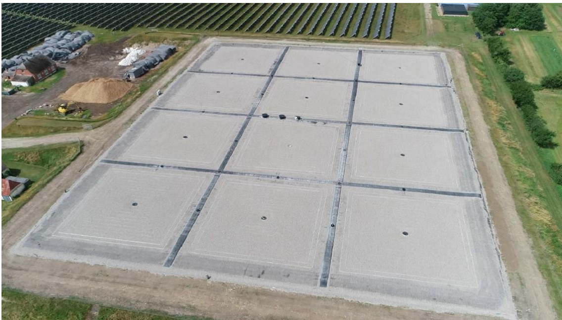
Figure 44: Aerial view of the new lid solution implemented in Marstal, displaying the 12 sub-sections 1 .
