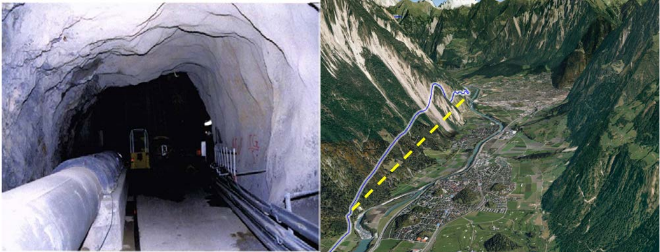
Figure 6.4.7: Typical gas pipeline inside tunnel and possible configuration in the area of Chur Village.
