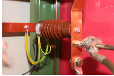
Fig. 4.2 Medium-voltage transducer installed in the primary substation of the tested network.
