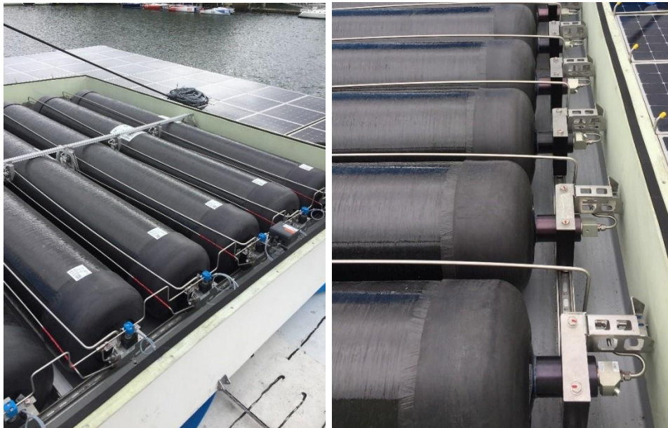
Figure 26: Type IV Hexagon Lincoln hydrogen cylinders, fixation and piping (3 TPRD outputs are visible with a yellow cap at right)
