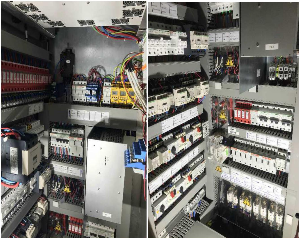
Figure 32: View of power cabinet (power distribution 400Vdc, left and 230Vac, right)
