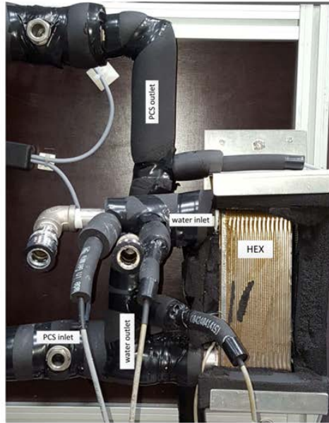
Figure 41: Side view of the installed heat exchanger in the final test-rig. For a better orientation, the front insulation has been removed.
