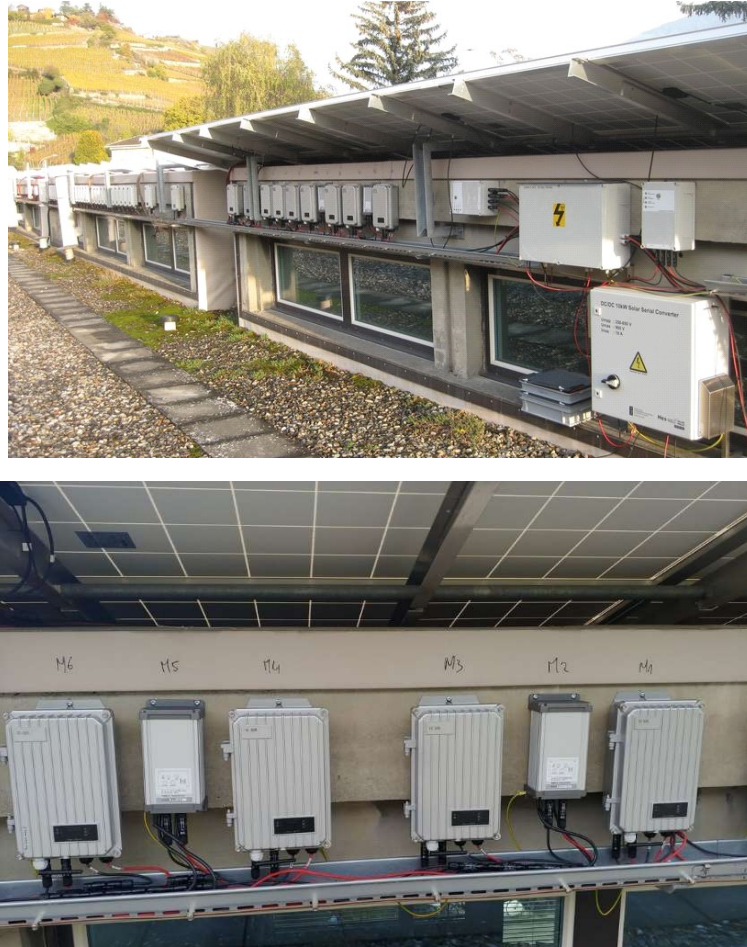
Figure 9: above: all DC/DC converters installed during the upgrade, the large converter for an entire string is installed at the very right end of the line, lower than the others. Below: The new DC/DC converters designed by Imperix (e.g. the small boxes, second and 5th in the row, counted from the left) during this project show a clear gain in size compared to the larger DC/DC converters of the previous generation (the 4 larger boxes).
