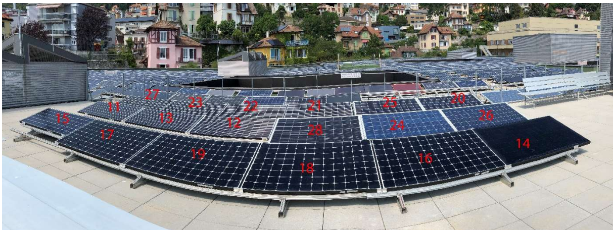
Figure 7: PV installation connected to the DC-bus system at EPFL-PV-lab, Neuchâtel.
