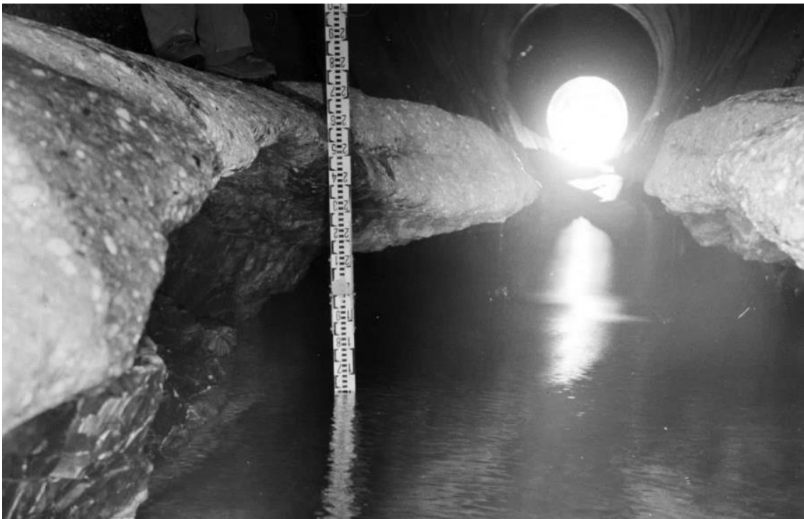
Figure 1: Invert damages at the Palagnedra SBT (Canton Ticino, Switzerland) after an exceptional flood event in 1978 (IM Maggia Engineering AG)
