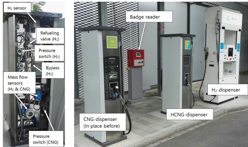
Fig. 29 Main components of the self-developed HCNG dispenser (left) and the refueling station at the move demonstration plant (right)
