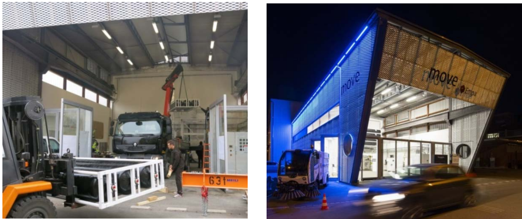
Fig. 3 Installation of the rack mounted end storage tanks onto the steel framework (left) and the demonstration plants exterior view by night (right)
