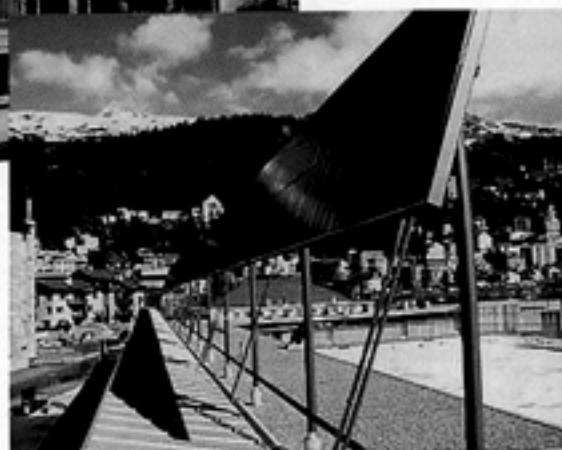
PV-Anlage in St. Moritz (OS/Photo TISO).
