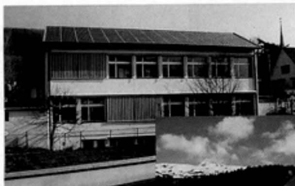
PV-Dachanlage in Wettingen (Photo NET AG).
