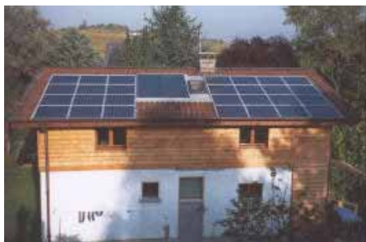
Marc Hottinger 3.24 kWp
