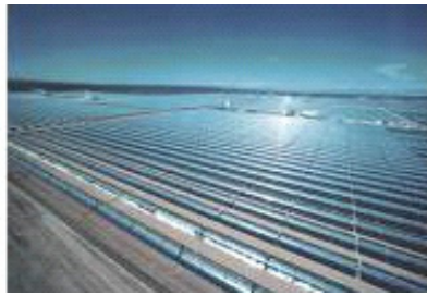
KJC, Kramer Junction, USA
