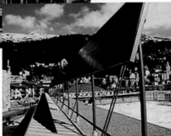
PV-Anlage in St. Moritz (OS/Photo TISO).
