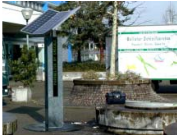
Figur 27: Autonomer Photovoltaik Obelisk Zürich (Bildquelle Enecolo)
