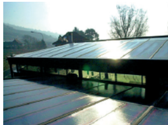
Figur 21: 5.5 kWp Dachintegration Freestyle (Bildquelle Solstis)
