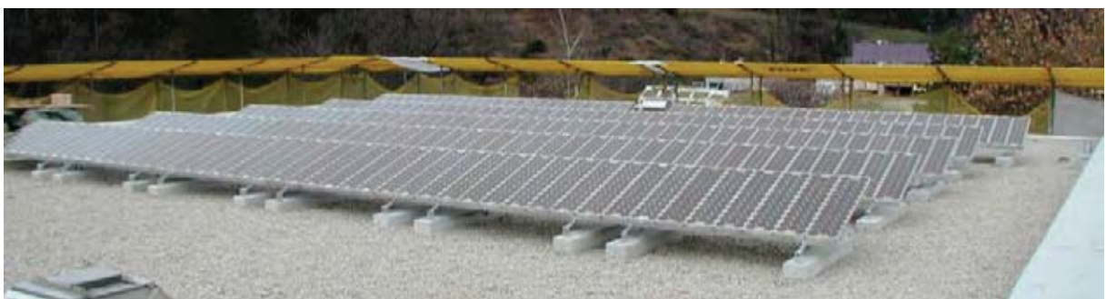
Figure : TISO 10kW -1982 - power plant on the new roof location in Trevano.
