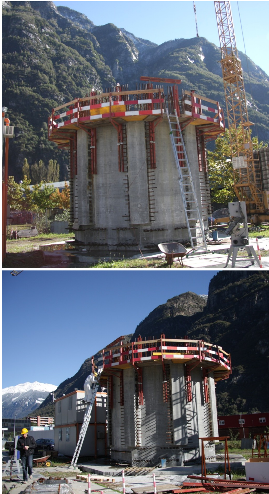
FIGURE 5: EXTERNAL VIEW OF THE NEW STORAGE PROTOTYPE.
