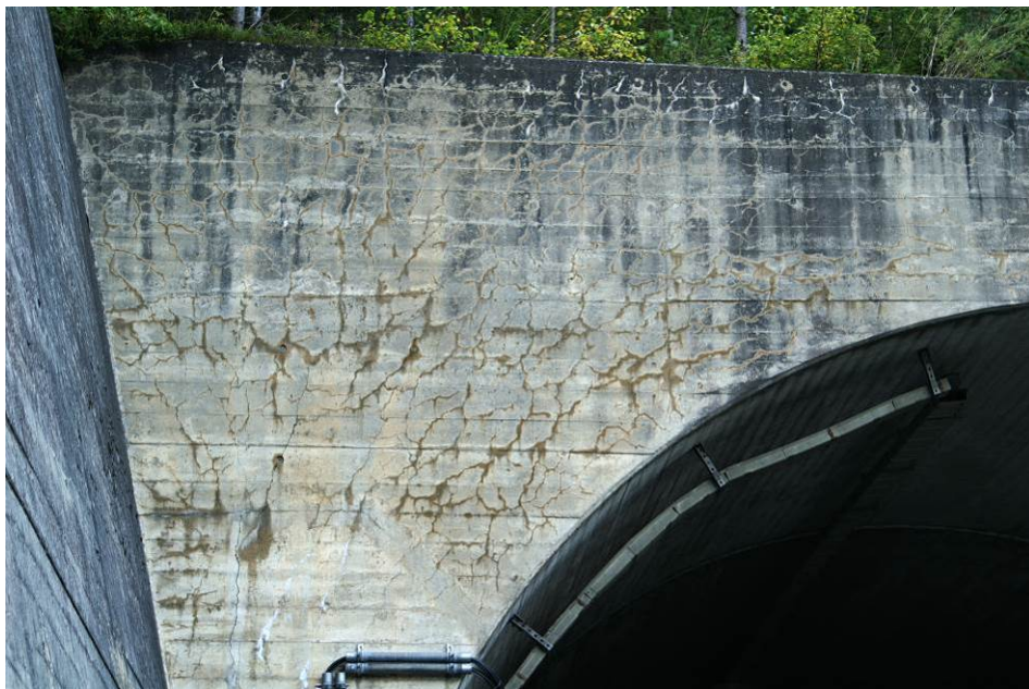
Figure 3.3: Dark-rimmed cracks showing a preferred orientation parallel to the compressive stress at the entrance of a tunnel.
