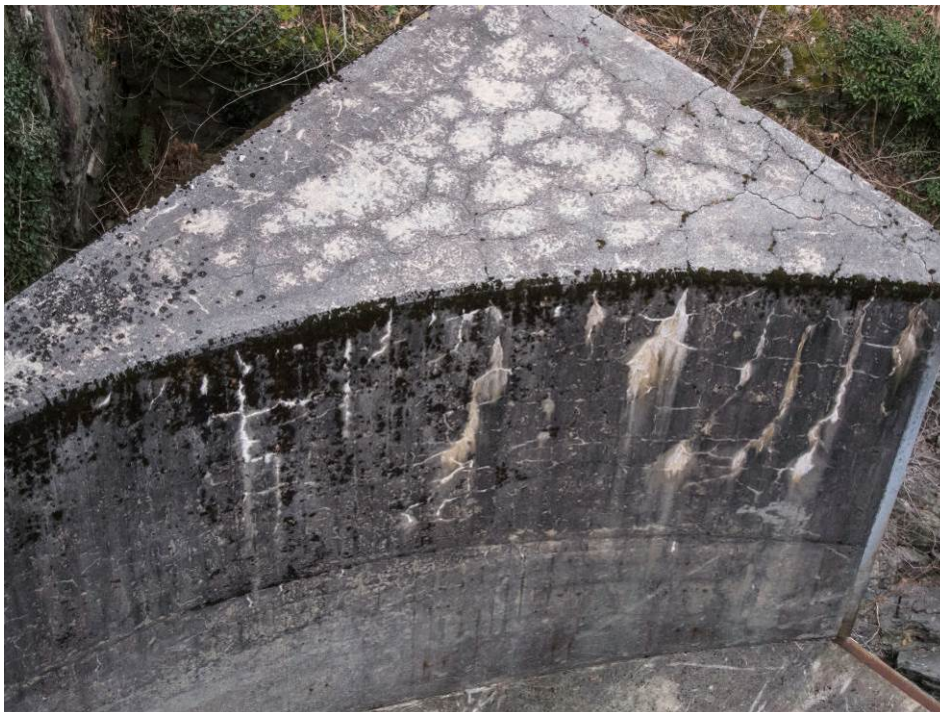
Figure 3.1: Cracks at the outlet of an overflow.
