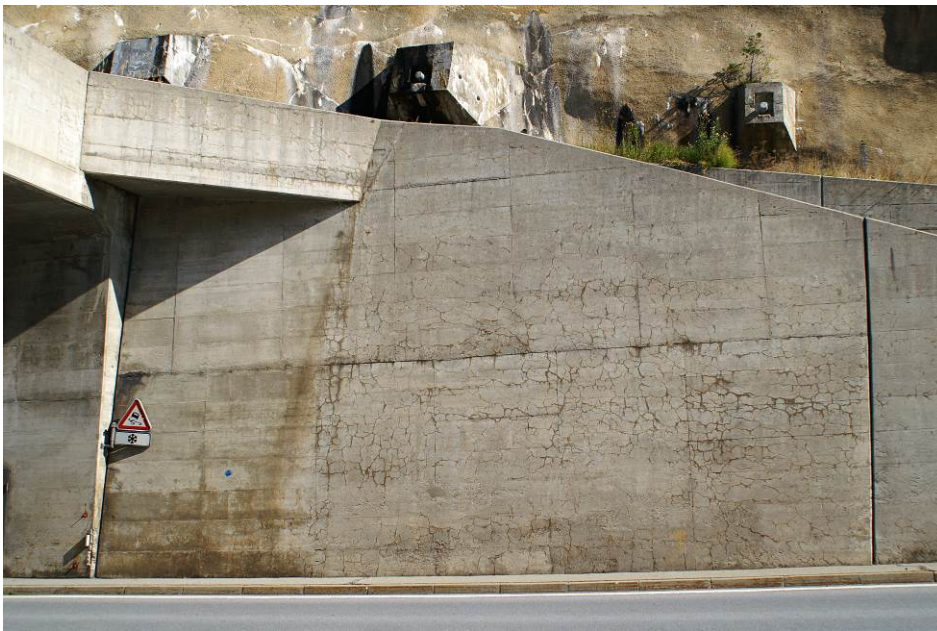
Figure 3.5: Supporting wall at the entrance of a gallery. Cracks lines with darkish deposits in the area exposed to rain and without deposits in the sheltered area.
