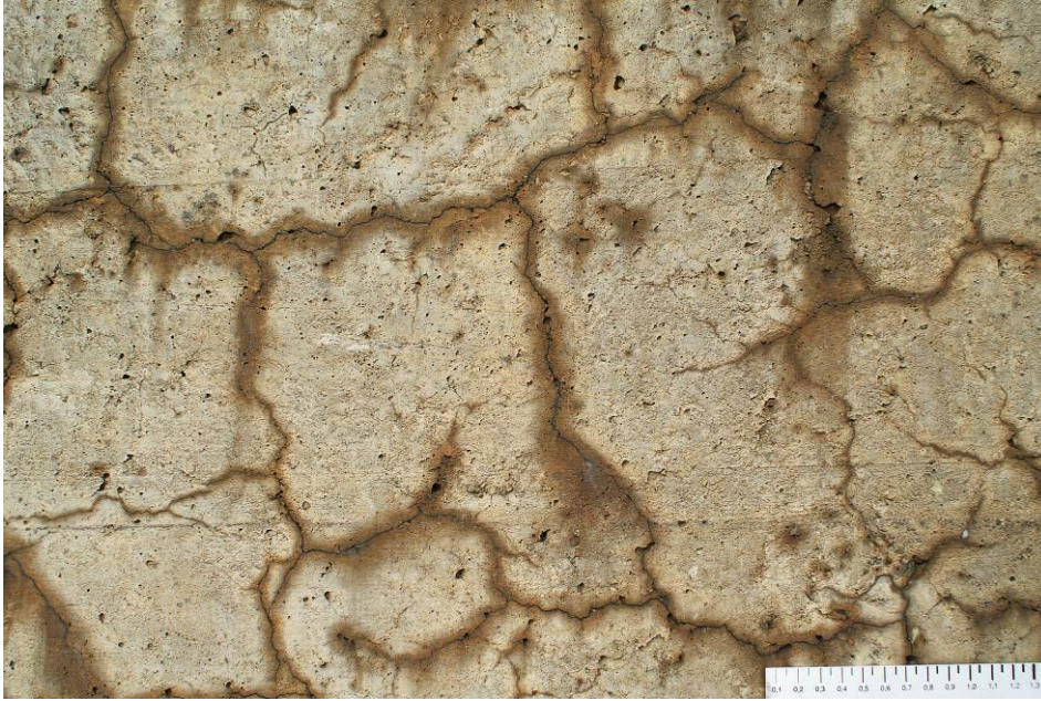
Figure 3.4: Cracks in a supporting wall lined with darkish deposits.
