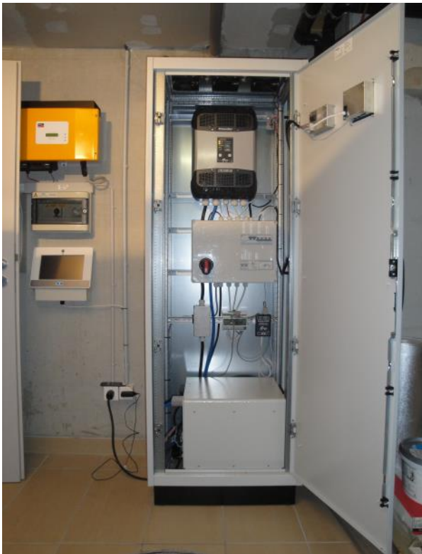
Figure 36: Battery-to-grid system installed in the households
