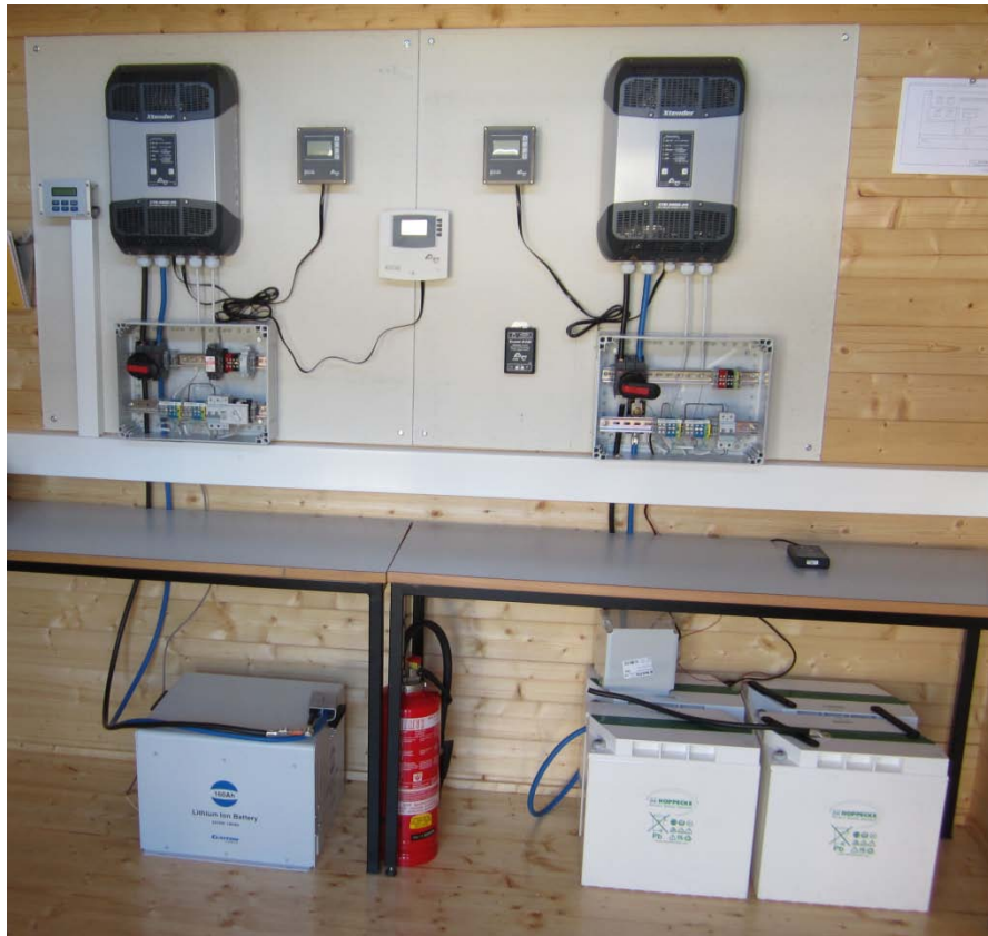
Figure 9 – S2G-Home, detail of the battery systems
