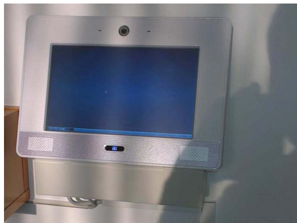
Figure 5 – Example of a touch panel installation
