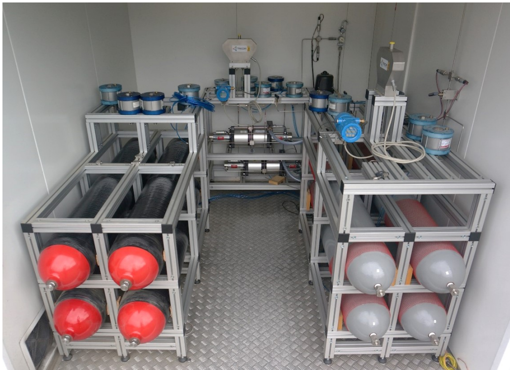
Figure 16 - Hydrogen refilling station container with cascade system
