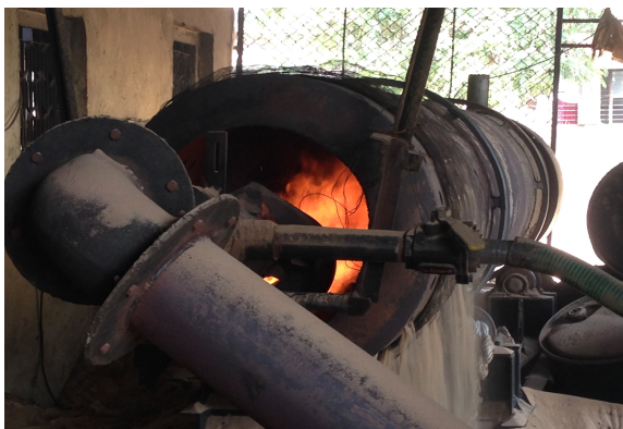
Figure 3: Thermal Gasifier for sand drying
