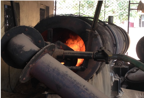
Figure 3: Thermal Gasifier for sand drying
