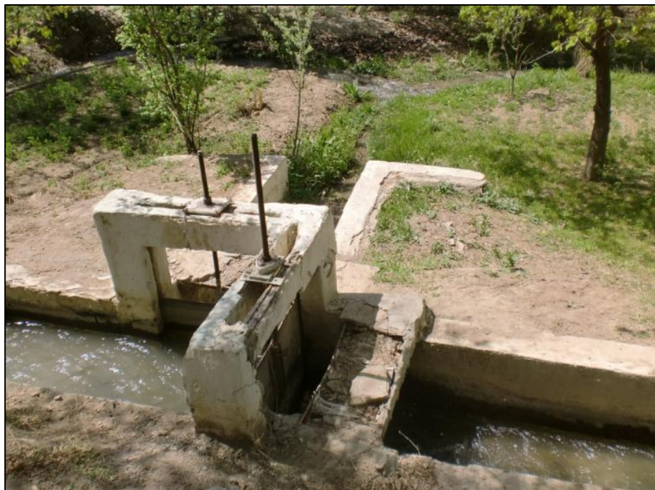
Dysfunctional secondary canal gate in Spitamen
