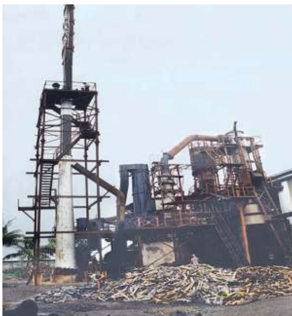
Demo DBC plant at Howrah
