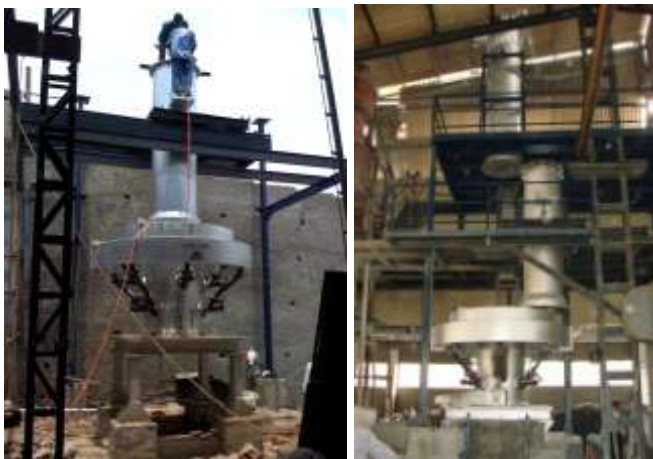
Split design 18-inch DBC at Ahmedabad
