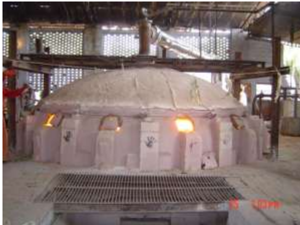
Recuperative pot furnace system
