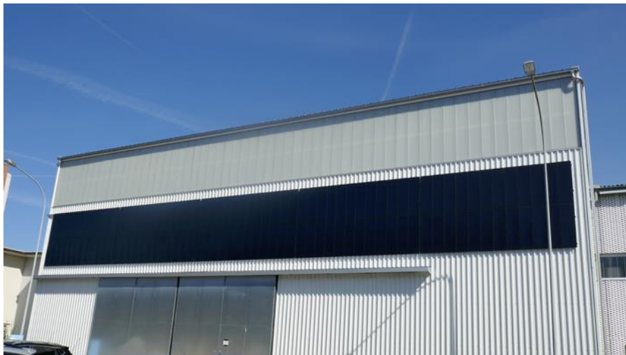
Figure 30 5kW facade installation with Flisom modules
