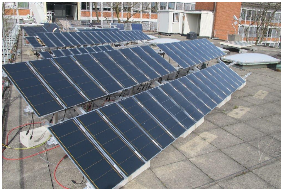
Figure 2 1kW Outdoor Installation in Dübendorf
