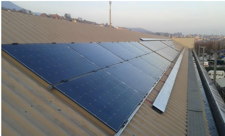
Figure 3.2: Four 3 kW p demonstration systems installed on the Innoparc building in Hauterive (NE). In the foreground are frameless Gen 2 and Gen 3 modules connected in November 2016.
