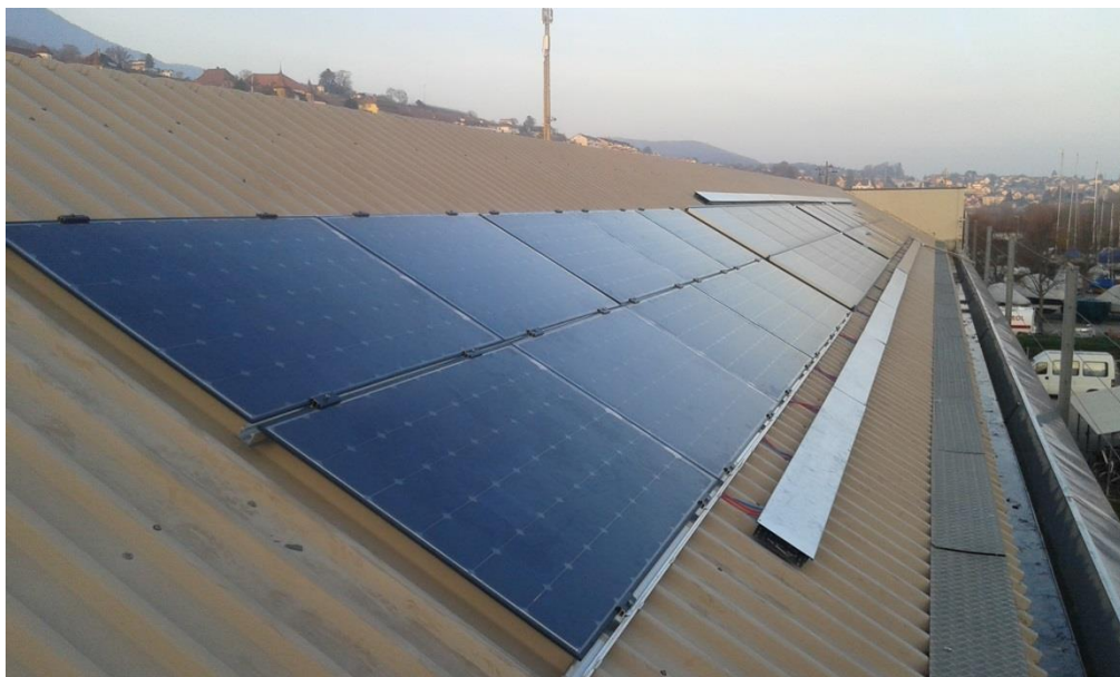
Figure 1.23: outdoor installation of 40 module, 10 reference and 30 modules produced within the Swiss Inno-HJT project
