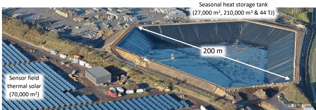
Figure 60: Fields of solar thermal collectors for district heating in Vojens, Denmark, (70,000 m 2 ) next to the seasonal storage tank (210,000 m 3 ) under construction in 2014-15 (still without the insulating and floating cover). (source: http://solarheateurope.eu/2020/05/19/vojens-district-heating/ )
