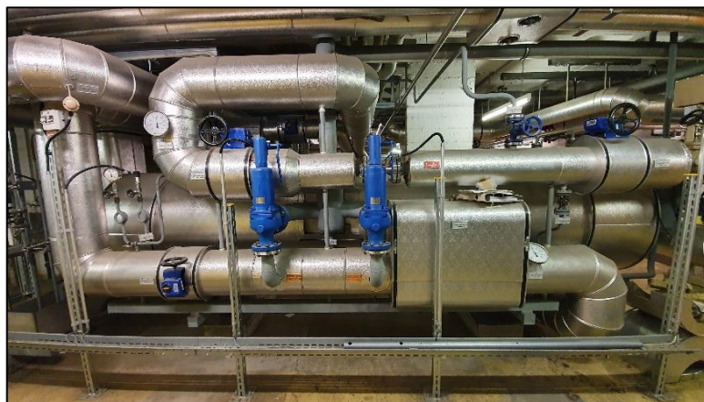
Figure 26 - Main substation feeding an old district heating of neighborhood.
