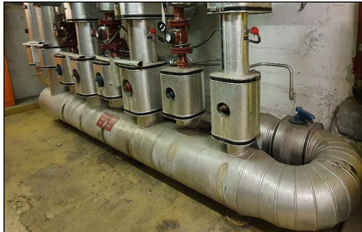
Figure 27 - Manifold with partially open bypass on the right.
