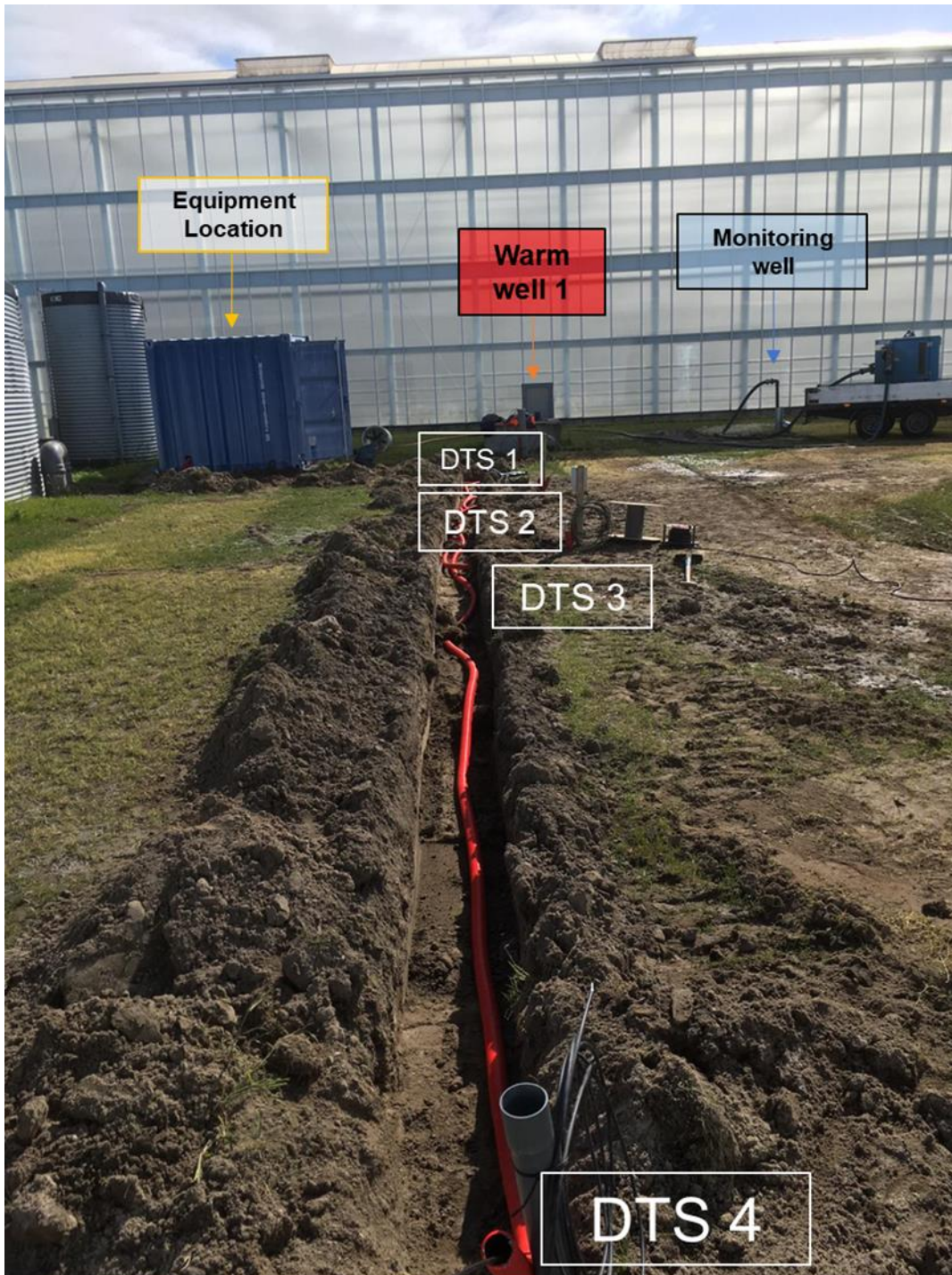
Figure 6: Overview of the monitoring facilities around ‘warm well 1’. New locations (Sept 2019) are: DTS 2 (deep), DTS 3 (deep) and the monitoring well. (When compared to figure 4, the viewpoint is from right to left).
